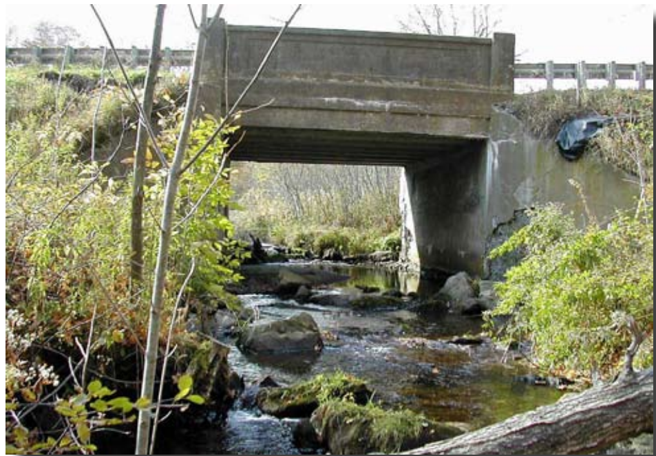
Figure 1.22—This box culvert has a concrete floor and no shallow edges for crawling-species passage. Photo: Scott Jackson, University of Massachusetts.
