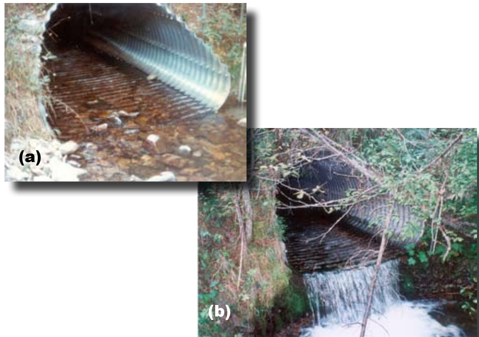
Figure 1.17—High-velocity discharge from undersized culverts causes downstream scour. (a) Culvert was placed at grade in 1979. (b) By 1998, undersized culvert had caused over 1 foot of downstream scour.
