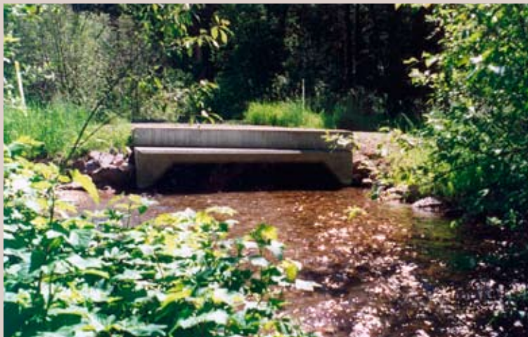
Figure 4.8—Brewster Creek road replacement box culvert, filled to 85 percent of its rise after 1 year.
