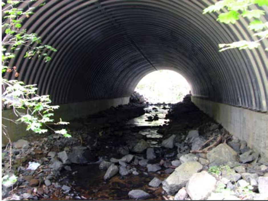
Figure 8.3—Results of a survey error. Footings were constructed 2 feet higher than the designed location because of a construction survey error. Always doublecheck surveys!
