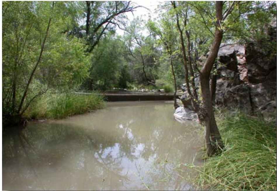
Figure 1.20—Elevated concrete-slab ford eliminates aquatic habitat area directly underneath the structure and blocks fish passage at low flows. However, it may not significantly alter the character of aquatic habitats upstream and downstream.
