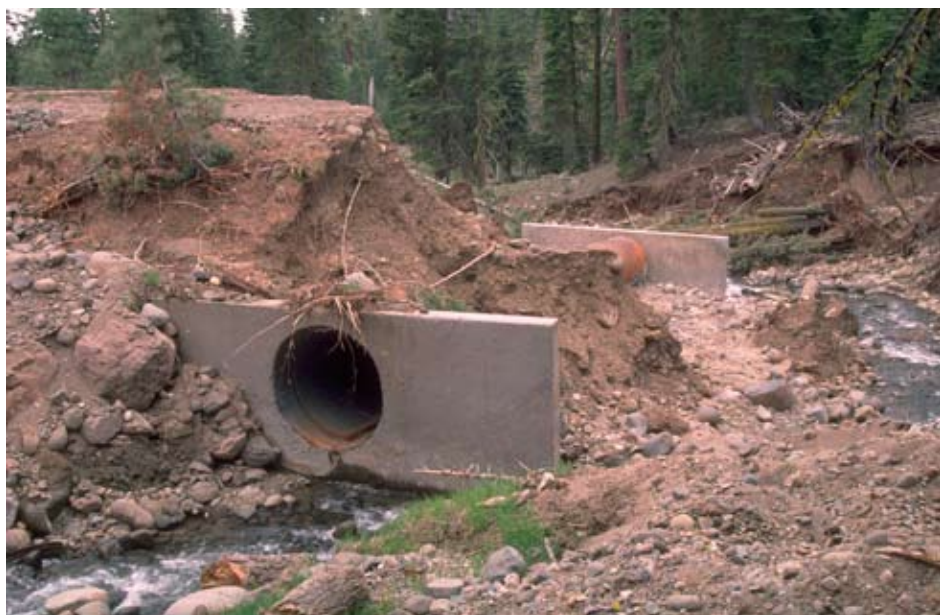
Figure 1.18—Culvert-crossing failure after flooding, Plumas National Forest, California.
