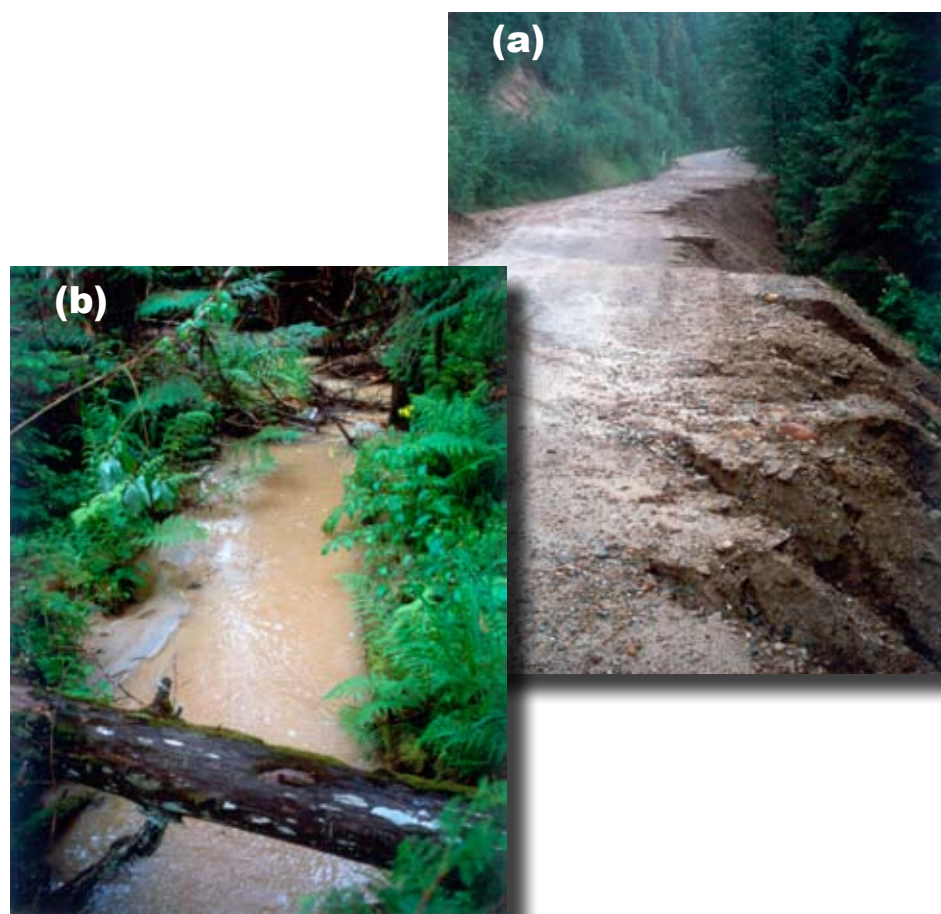
Figure 4.2—Flood-damage surveys can provide historical context for stream condition. (a) On Gap Creek in northeastern Washington, extensive erosion occurred on a riparian road in unconsolidated glacial sands during a 1993 flood. (b) Sediment filled the channel for several years but this transport channel remained stable and the sediment progressively cleared out during subsequent high flows.
