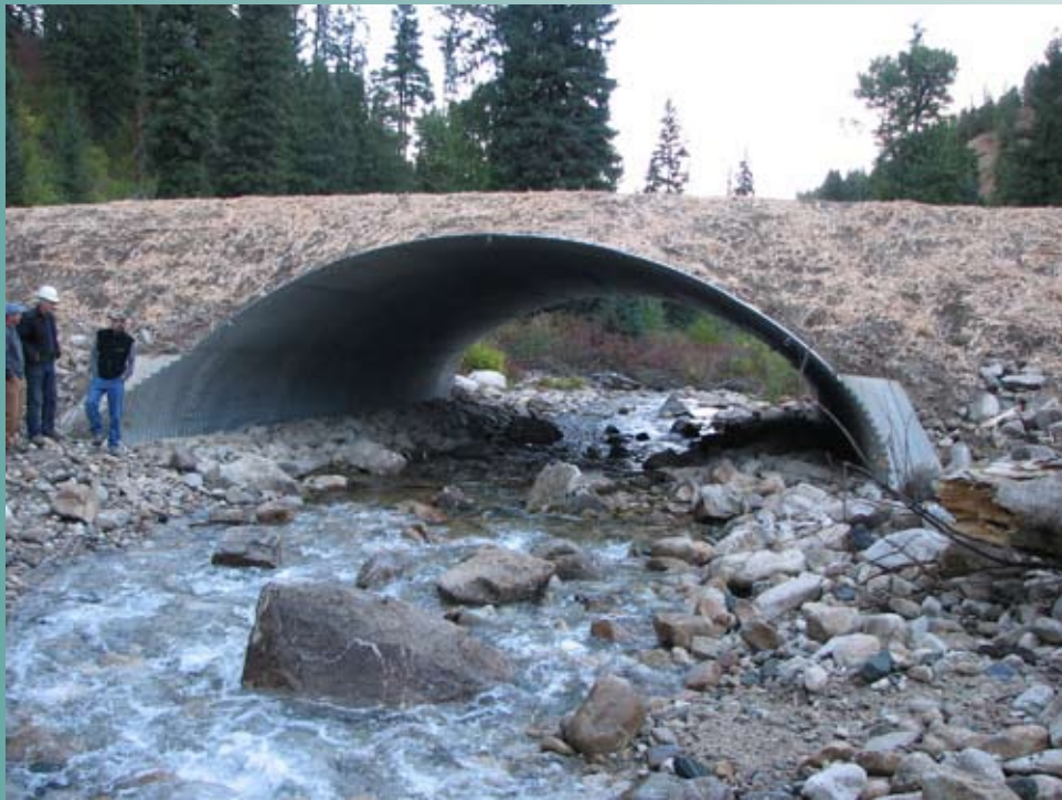
Figure 3.1—Roaring River crossing site before-and-after culvert replacement in 2007, Boise National Forest, Idaho.
