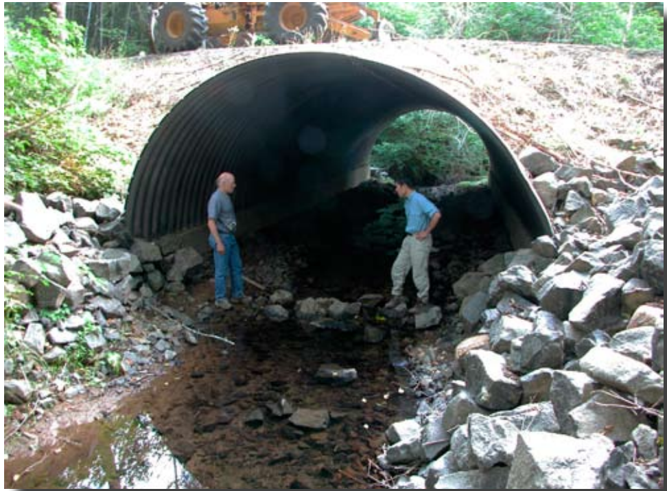
Figure 8.11—Example of uneven backfill and compaction. The right side was backfilled before the left side instead of even lifts on both sides, causing the distortion visible in this photo. The distortion induces eccentric loadings on the footings, as well as bending stresses at the anchor bolts on both footings.
