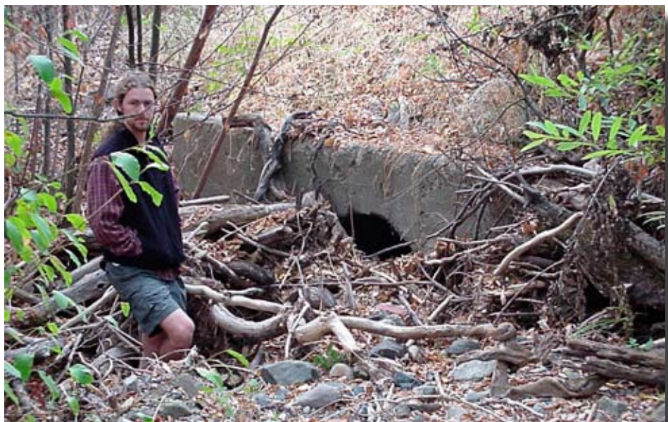
Figure 1.16—Debris and sediment at culvert inlet can be a fish barrier. Photo courtesy of Ross Taylor and Associates, McKinleyville, California.
