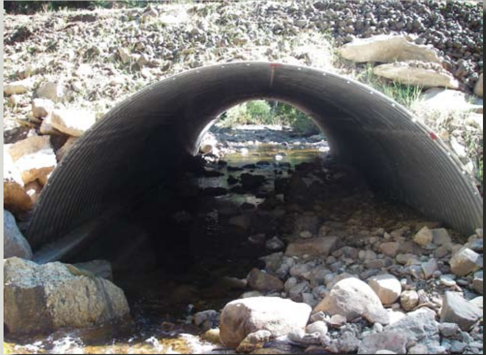
Figure 8.2—Open-bottom arch stream-simulation culvert on Wilson Creek, Boise National Forest, Idaho.
