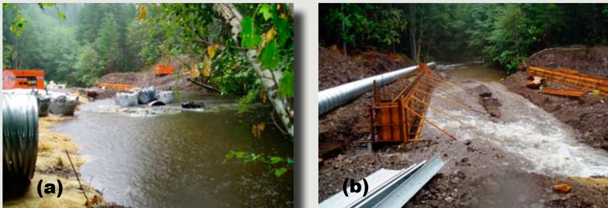
Figure 8.9—Unusual summer storm overwhelms bypass system. (a) Looking downstream at bypass pipe, now in mid-channel. (b) Looking downstream through the open excavation.
