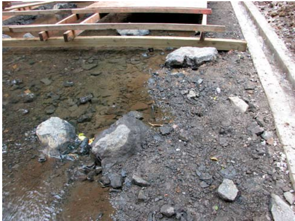
Figure 8.14—Newly constructed stream-simulation bed for a bottomless arch. The stream-simulation bed material is manufactured rock from a commercial source. Footing backfill and stream-simulation bed material were backfilled and compacted at the same time. Placing the stream-simulation bed is much easier before the structure is in place.
