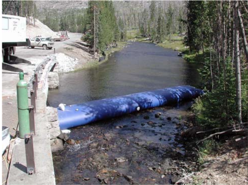
Figure 2.6—Isolating the construction area at a bridge reconstruction site in Yellowstone National Park. Photo: Dan Rhodes, National Park Service.
