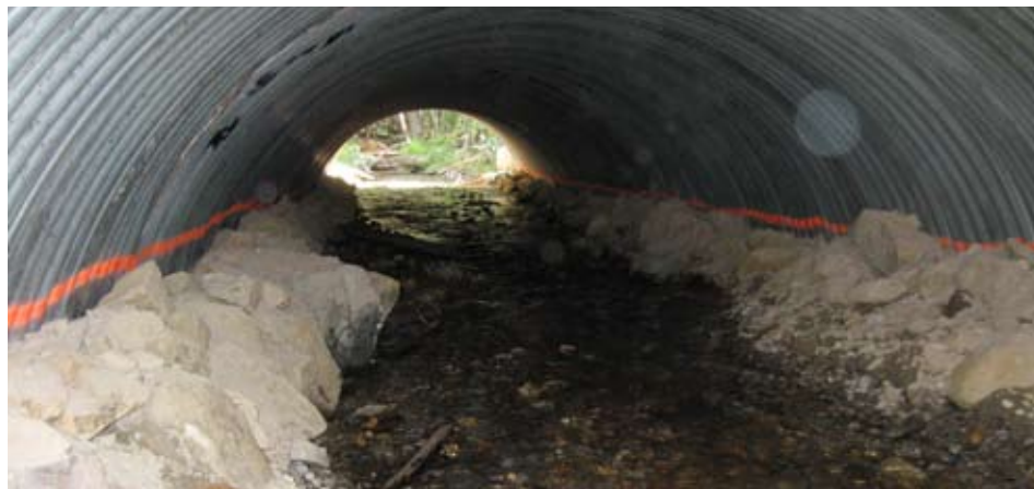
Figure 7.16—Newly constructed (2006) stream-simulation channel and banks, Surveyor Creek, Lolo National Forest, ID. The top of the bank is at bankfull elevation, indicated by the painted line. Note the transition between natural banks outside and constructed banks inside the culvert.
