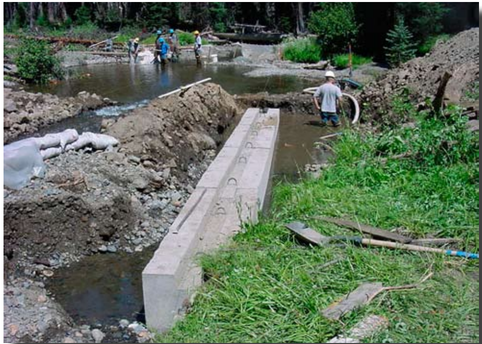
Figure G.10—South Fork Desolation Creek looking upstream. The crew captured fish trapped within the construction area as the foundation trenches were dewatered.
